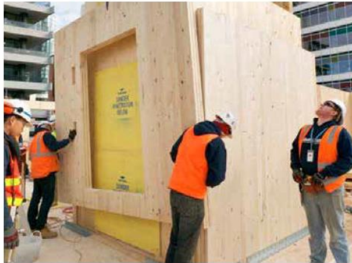
Up she goes .. construction starts on the CLT Forte building in Melbourne.
